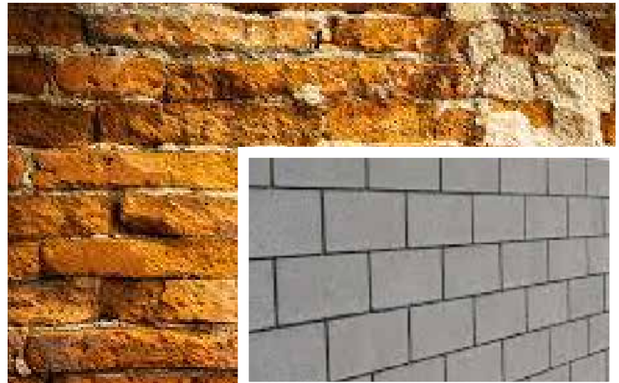
Comparison view of Clay Bricks and HCIL Solid Bricks after a few years. The traditional clay brick damages within 15-20 years where HCIL Solid bricks can survive upto 100 years.
